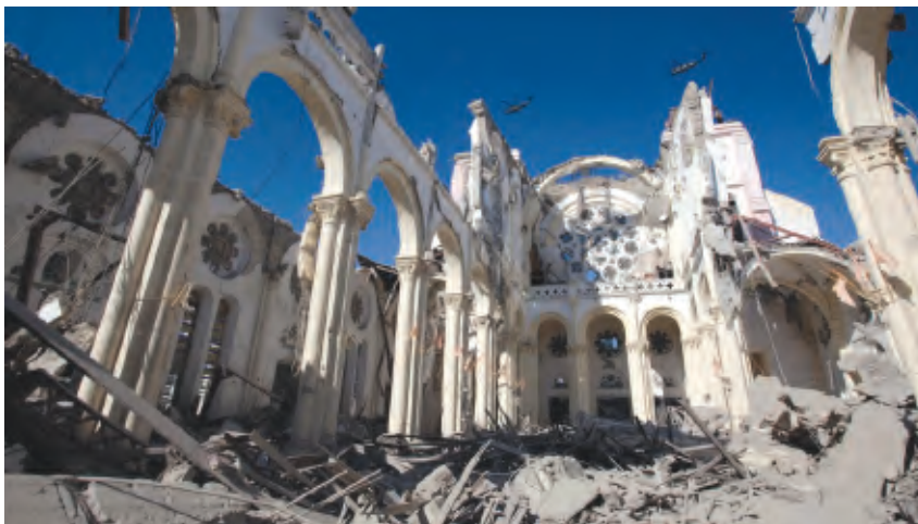
Cathedral of Our Lady of the Assumption, destroyed in the earthquake. All that remained intact was the statue of Christ on the Cross (see front cover).
